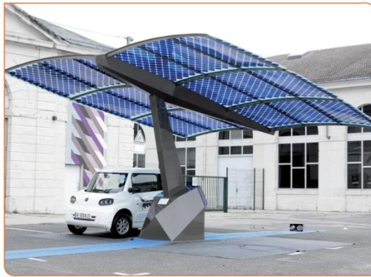
The SUDI shadow screen (a true photovoltaic charging station for electric cars)
